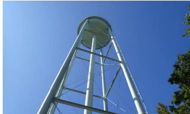
Photo 1 Towers are subjected to weather extremes and should be inspected approximately every 8 to ten years.
