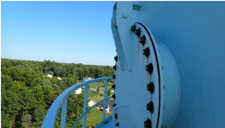
Photo 2 The inspection process look at all features on a water storage tank, such as manways and railings.
